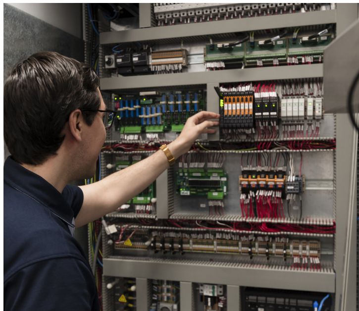
ATC-E TEST STATION
