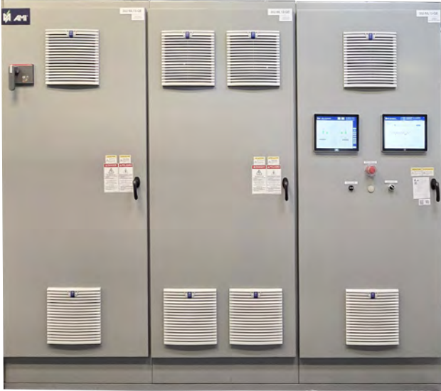
DIGIQUAD™ CONTROL CABINET FRONT VIEW
