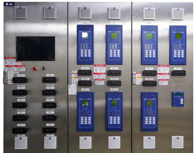
DIGISVC® FCR CONTROL CABINET FRONT VIEW
