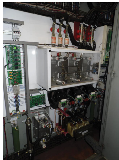
Figure 9. Field Power Supply Cabinet
