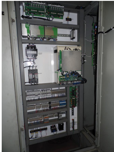
Figure 6. Armature Bridge Current Control Cabinet
