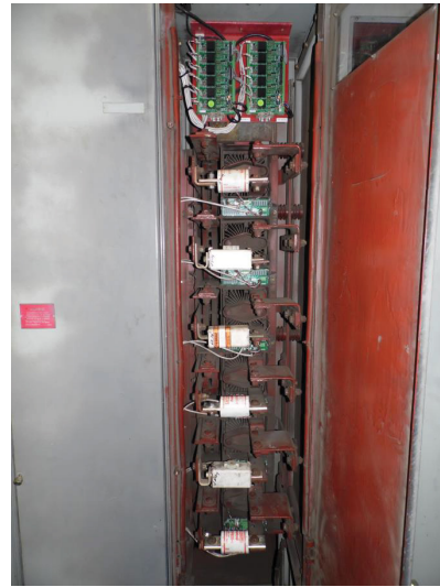
Figure 7. SCR Cabinet Installation
