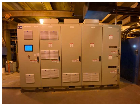
Fig. 5 – 7.2kV 3MVA MV AC Valve Cabinet
