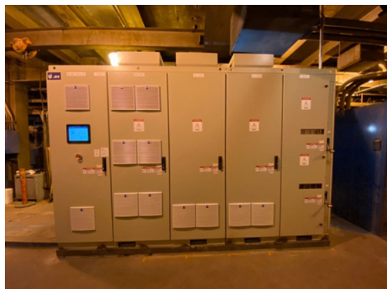
Fig. 5 – 7.2kV 3MVA MV AC Valve Cabinet
